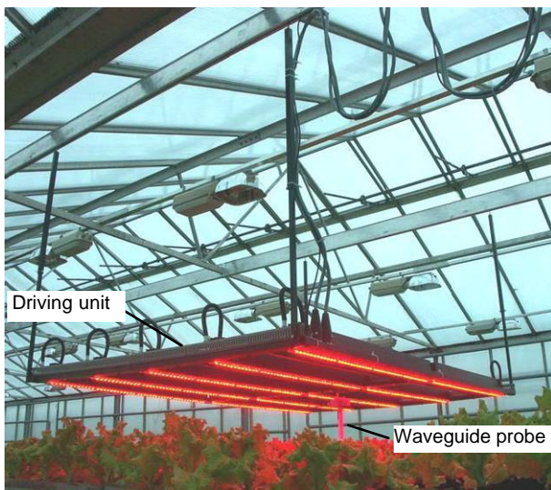
Fig. 4. Solid-state illuminator installed in the greenhouse
