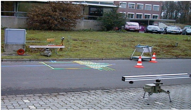
Fig. 15. Measuring disposition and equipment
