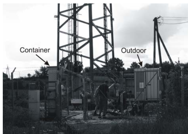
Fig. 1. Overall view of the radio base station
