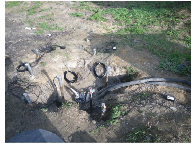
Fig. 3. Physical installation of the temperature probes at the area.
