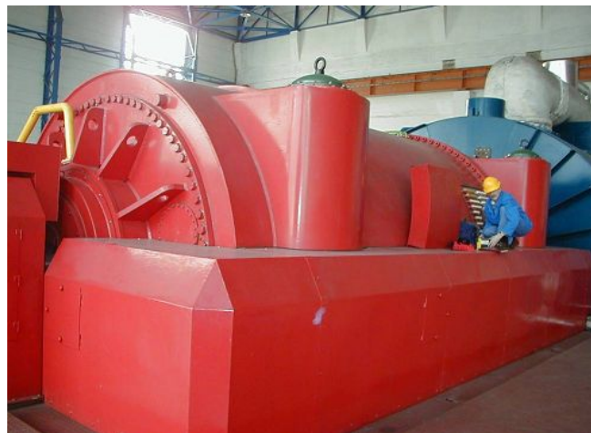
Fig. 1. Synchronous turbogenerator in TPP Plomin2.
