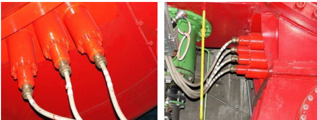
Fig. 3. Signal cable glands.
