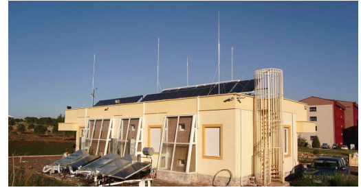
Fig. 5. Solar trackers with air termination rods.
