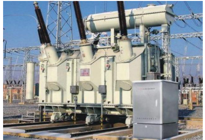
Fig. 2. Sample DGA data gathering for the online chromatographic monitoring system of transformers [95].
