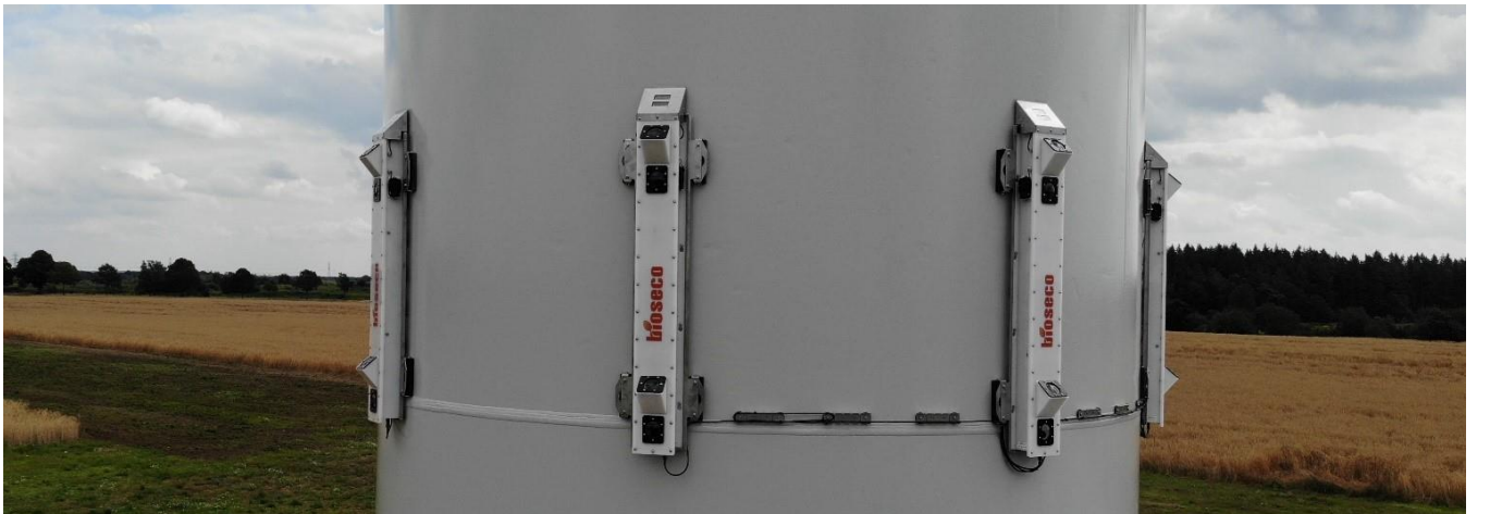
Fig. 3. The Bioseco BPS long-range system at the test site used for system validation.
