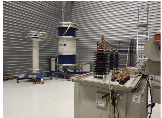
Fig. 6. Transformer during routine tests.
