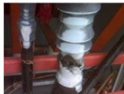
Fig. 3. High voltage underground cable termination fault.
