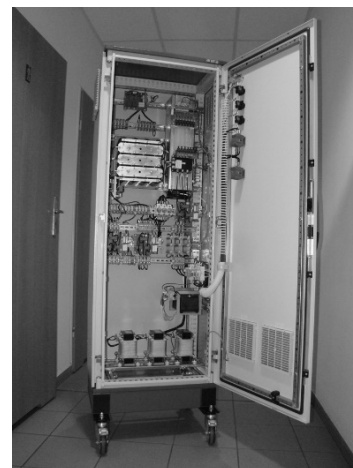
Fig. 4. View of the active power filter (APF) developed.
