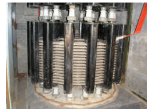
Fig. 1. Air electric reactor (phase "C")
