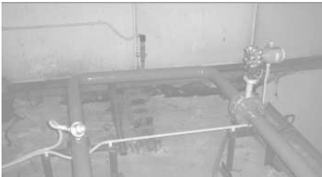
Fig. 5. Measurement of flow, temperature and pressure
