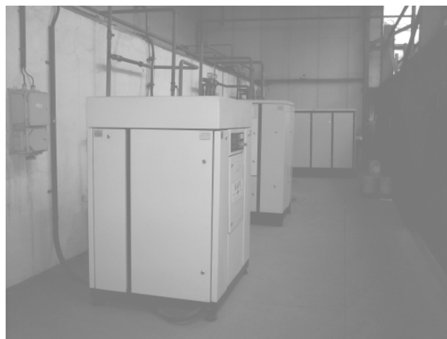
Fig. 1. View into compressor station
