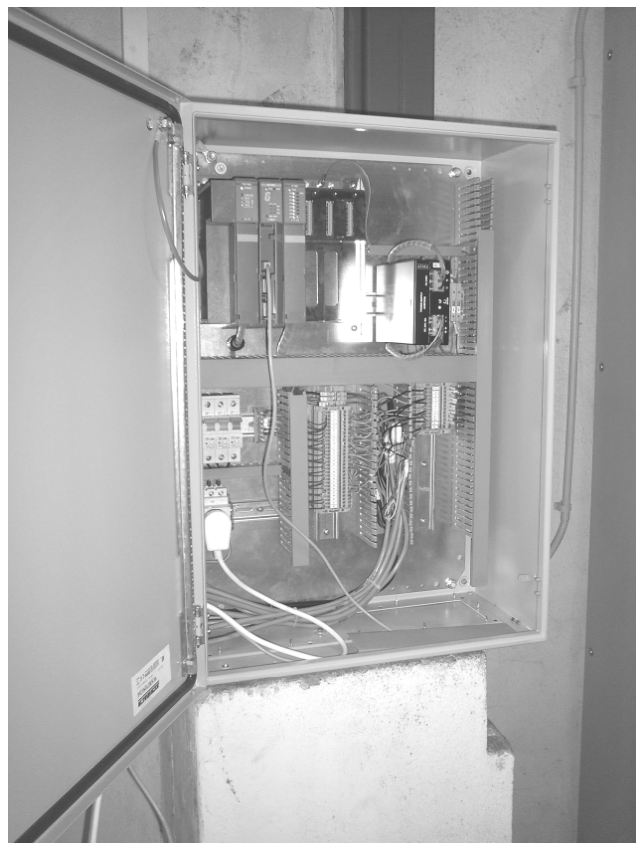
Fig. 4. View into switchboard
