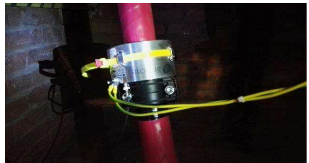
Fig. 5. Inductive couplers installed at point A.
