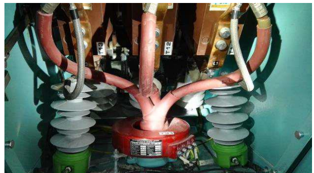
Fig. 4. Capacitive couplers installed at point A.
