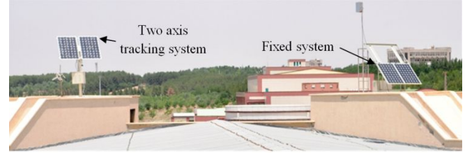
Fig. 9. View from the rooftop systems.
